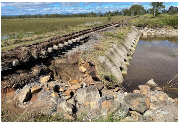
Figure 4 – Examples of Moura Coal System Initial Damage Assessment
