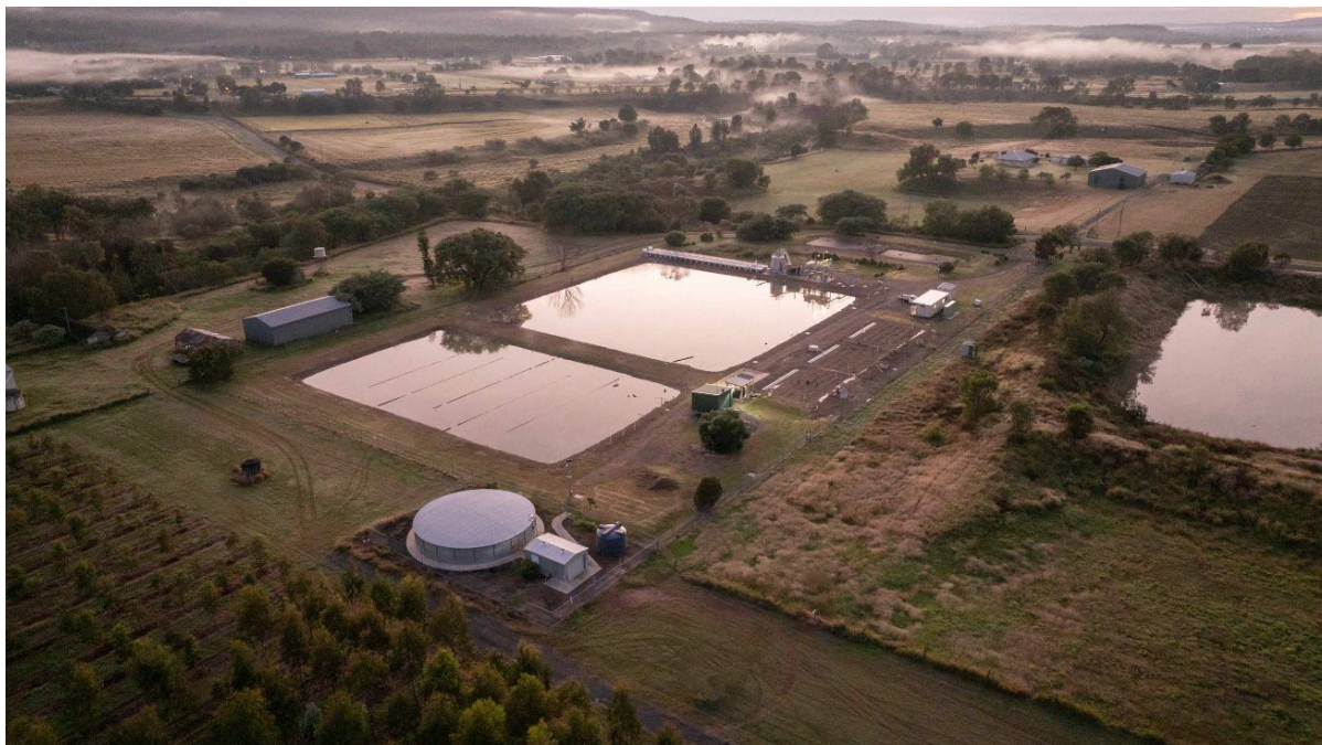
Figure 16 Helidon Wastewater Treatment Plant, Lockyer Valley Regional Council
