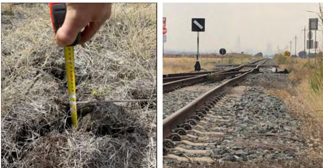
Figure 15 (Left) Ground Cracks (~400mm) next to formation in Callide branch. (Right) Poor track geometry at Dakenba 12 points.
