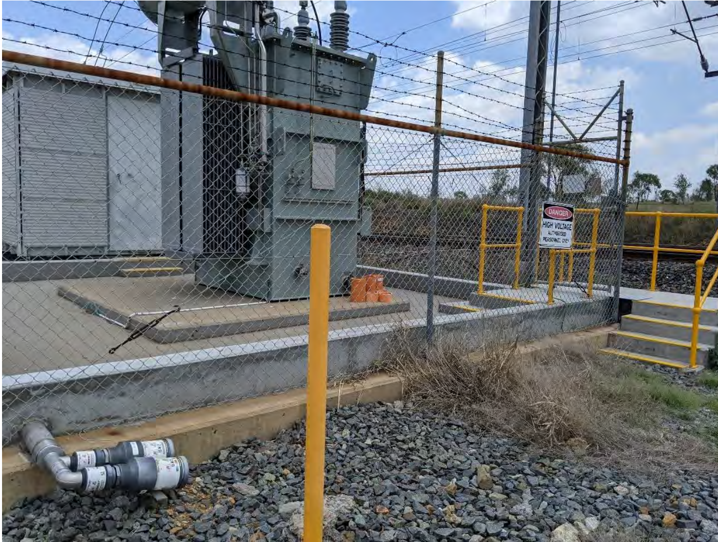
FIGURE 1 PROGRAM SEEKS TO RENEW PRIORITY ELECTRICAL ASSETS TO MAINTAIN SERVICE RELIABILITY. THE SPARE AUTO AND TRANSFORMER & BUND RENEWAL IN WINDAH WAS PART OF THE FY20 CLAIM. THIS WAS PROTECTED WITH BARBED WIRE FOR PUBLIC SAFETY (FIGURE 13) AND HAS A CHEMICAL SYSTEM WHICH FACTORED SPILLAGES FROM THE AUTO TRANSFORMER. A CHEMICAL SEPARATOR WAS INSTALLED TO ENSURE OIL WAS SEPARATED FROM WATER AS SHOWN IN THE FIGURE
