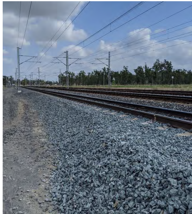
FIGURE 3 BLACKWATER NCL NEW LAID BALLAST (RM900 BALLAST UNDERCUTTING). THE BALLAST HAS A DISTINCTIVE BRIGHTER COLOUR WITH DISTINCT IRREGULAR SHAPING TO MAXIMISE “LOCKING” TOGETHER
