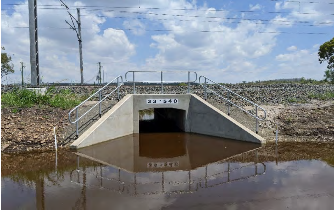
FIGURE 1 ONE OF THE PRIMARY OBJECTIVES FOR THE PROJECT IS TO REPAIR, REPLACE OR REMOVE LIFE – EXPIRED STRUCTURES ON THE CQCN, WITH NEW STRUCTURES COMPLAINT TO 300LA LOADING CONFIGURATION. THE ABOVE IS AN EXAMPLE OF A NEWLY CONSTRUCTED CULVERT INCORPORATING NEW STANDARDS TO HAVE HANDRAILS INSTALLED. DUE TO BLOCKAGE ON THE ACCESS ROAD NOT ALLOWING WATER TO DRAIN DOWN THE BANK WATER HAS POOLED AROUND THE STRUCTURE. AURIZON SITE STAFF IMMEDIATELY CONTACTED ENGINEERING TO REMOVE THE OBSTRUCTION AND ALLOW THE WATER TO DRAIN FROM THE ACCESS ROAD
