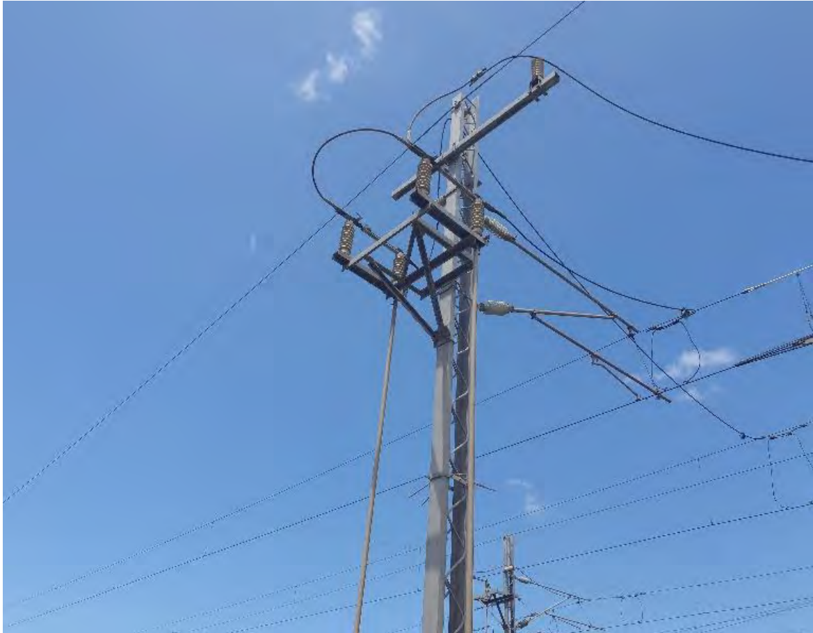
Figure 5-4 Replacement of clamps or arms is critical in maintaining a safe and operational network
