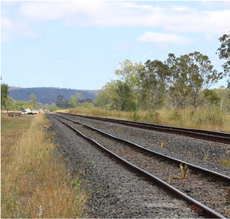
Figure 6.13. Formation failure R2J
