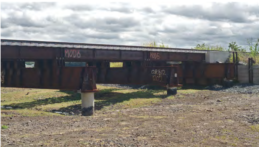
Figure 4.5. Steel bridge at kilometer 57.460km near Rosewood. Originally Queensland Rail planned to replace the timber bridge with a 30 tal concrete bridge; however, after considering Inland Rail installed a 20 tal steel bridge with a shorter life of 25 years.
