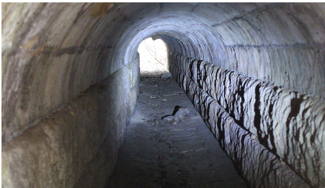
Figure 5.10. Original culvert installed in the late 1800s at approximately Kilometre 145.000 near Tunnel 2. At the far end maintenance issues with the roof of the culvert can be seen. This type of defect would require some method of lining to control.
