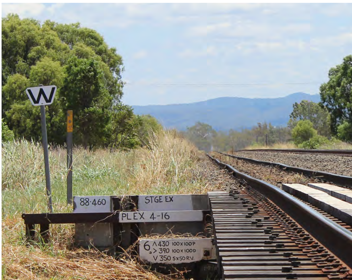
Figure 6.31. Failed formation R2J.
