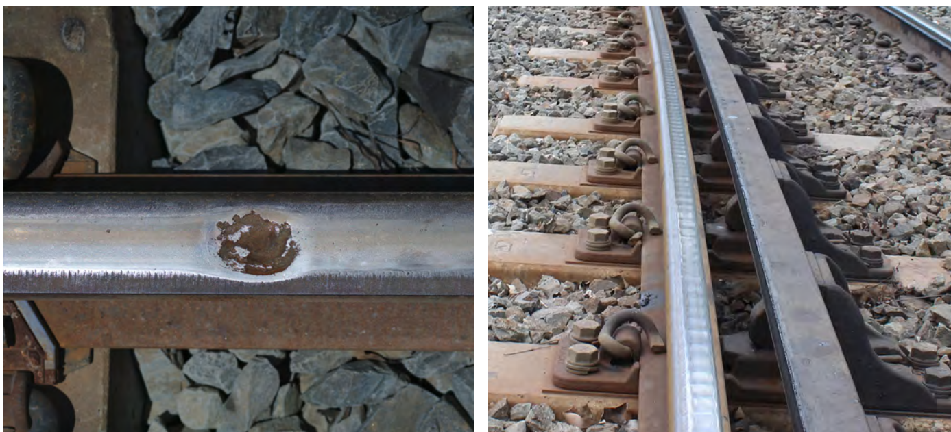
Figure 6.10. Rail defects; left photo shows a squat and right photo shows corrugations with a wavelength of approximately 50mm on the Toowoomba Range.
