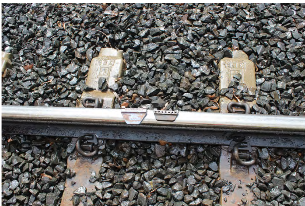
Figure 5.13. Location of proposed sleeper replacement on the Toowoomba Range. Current spacers used to manage gauge widening are placed on top of the rail. Evidence of movement of the rail is clear on the left hand pandrol clip.
