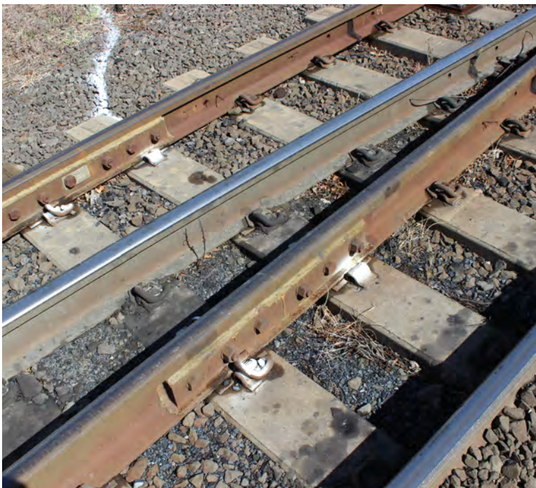
Figure 6.9 Sleeper and fastener defect
