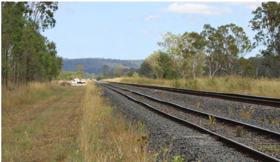
Figure 5.9. Top and line defect at Kilometre 65.300. SYSTRA Scott Lister was advised that this site was resurfaced approximately 3 months previously; a top and line defect so soon after resurfacing indicates potential formation rebuild is required.
