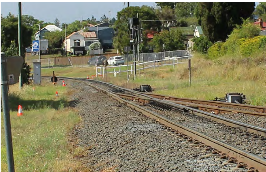
Figure 4.3. Failed formation site at Kilometre 160.395 in Toowoomba already identified by Queensland Rail as a site requiring formation rebuild.
