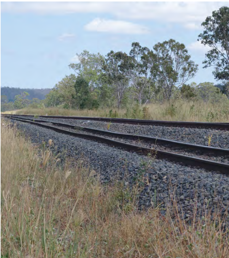
Figure 6.8. Track geometry defect
