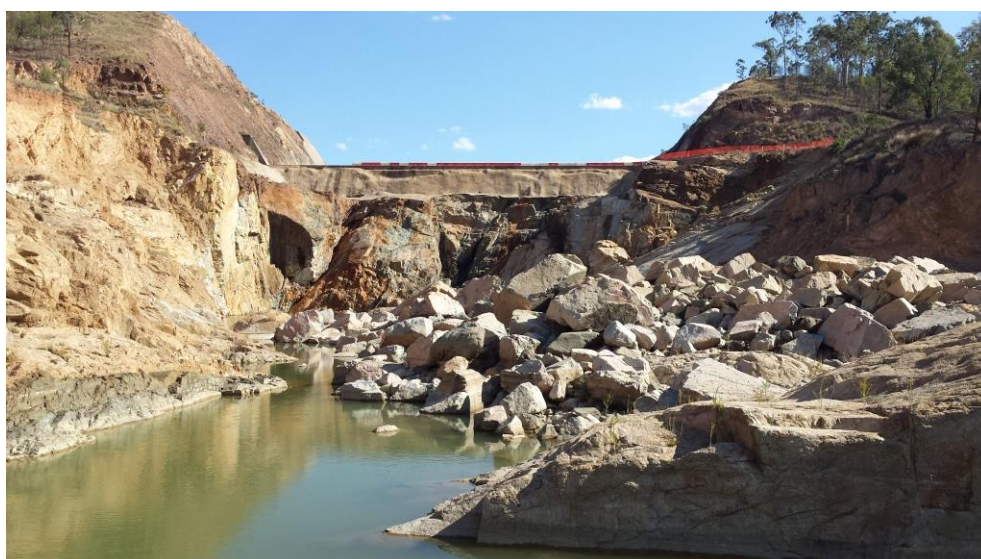
Figure 1.3: Flood damage to the Boondooma Dam spillway, 2013
