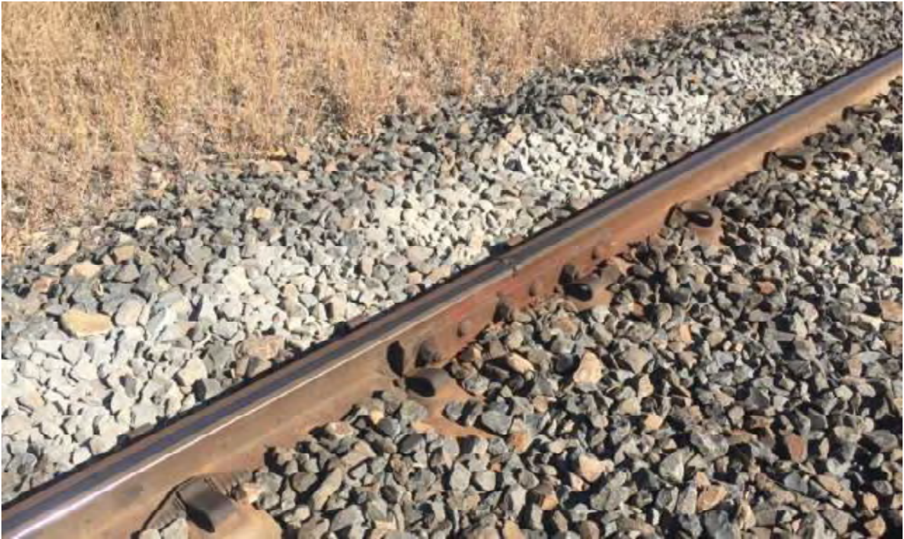
Figure 18 Battered and frozen joint
