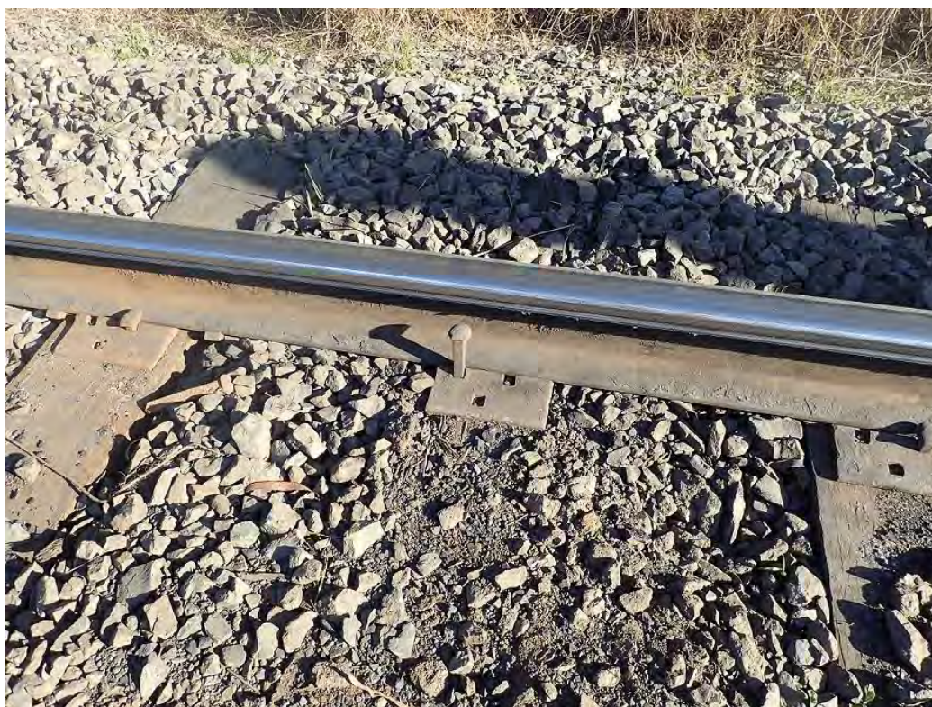
Figure 9: Deteriorated timber sleepers along the West Moreton network
