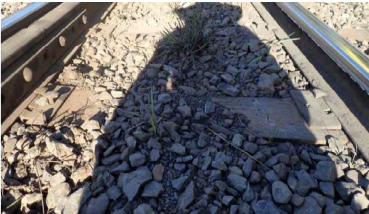
Figure 5: Poor formation issues and vegetation growing from track-bed
