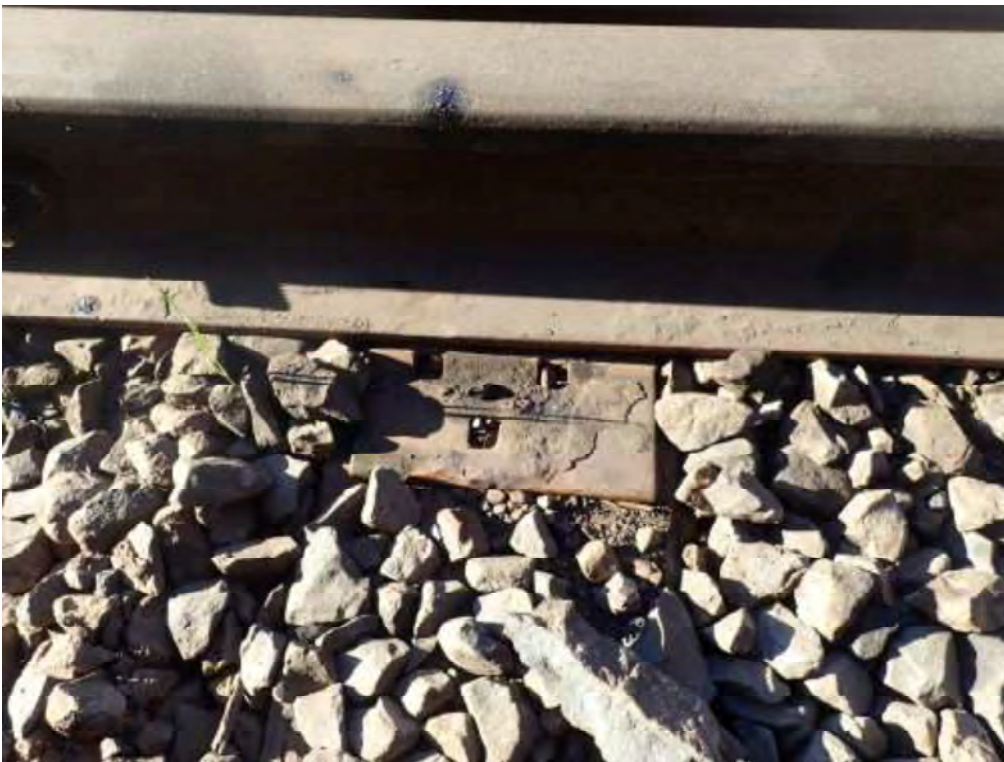
Figure 10: Missing dog spike
