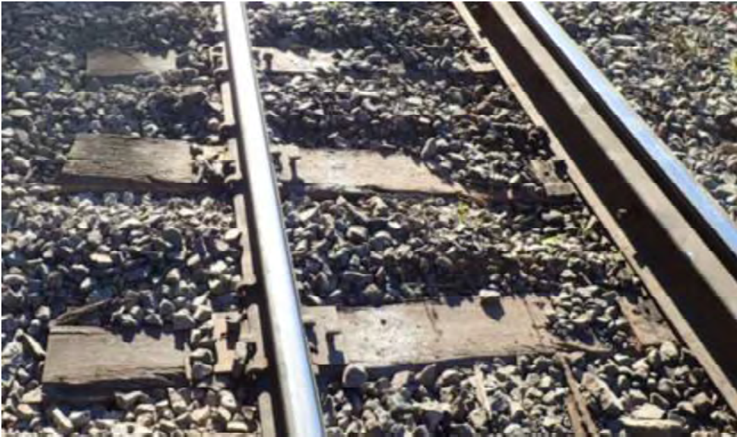
Figure 12: Skewed timber sleeper splintering
