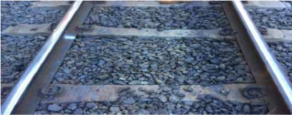
Figure 9: Skewed sleepers caused by excessive longitudinal forces
