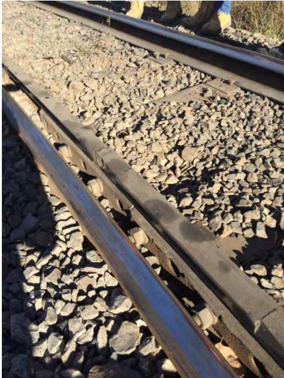
Figure 3: Poor formation conditions evidenced by the vegetation in the sleeper bays
