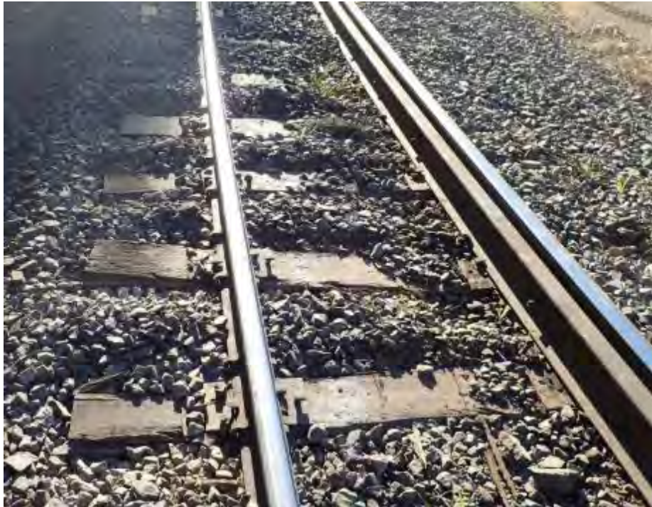
Figure 2: Areas in the West Moreton system needing Formation Repairs
