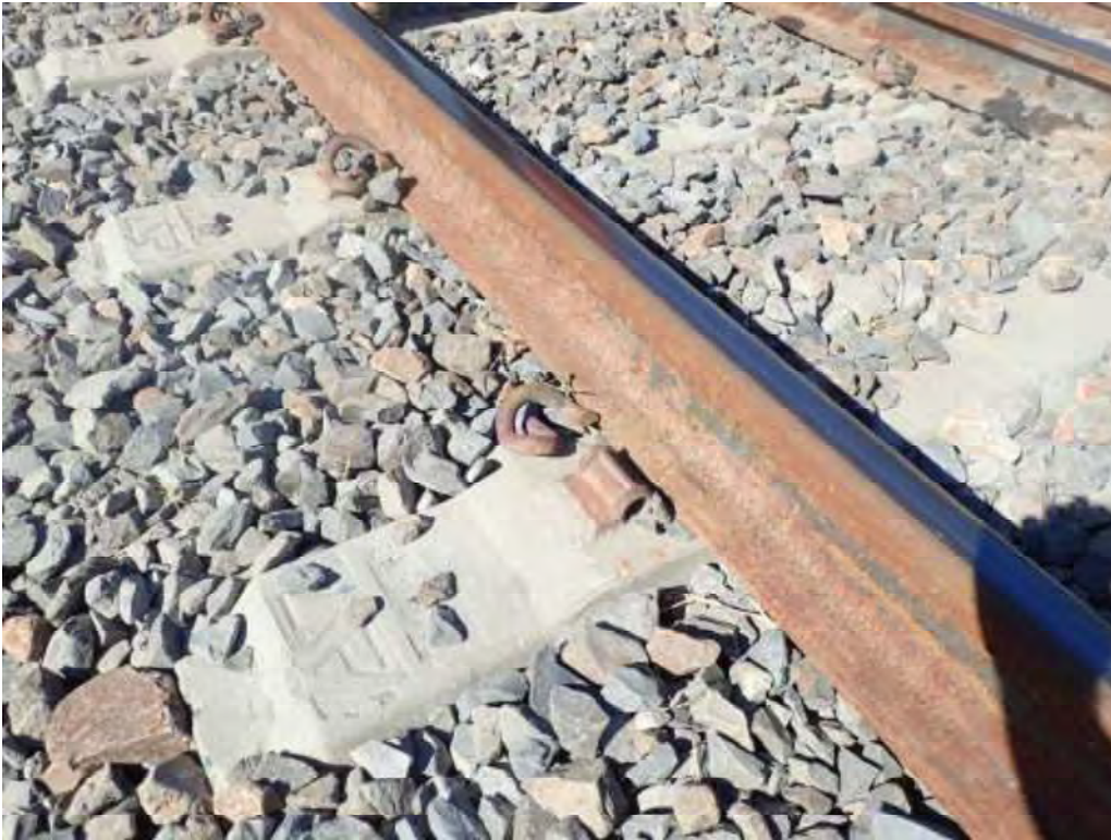
Figure 11: Missing sleeper clips and nylon
