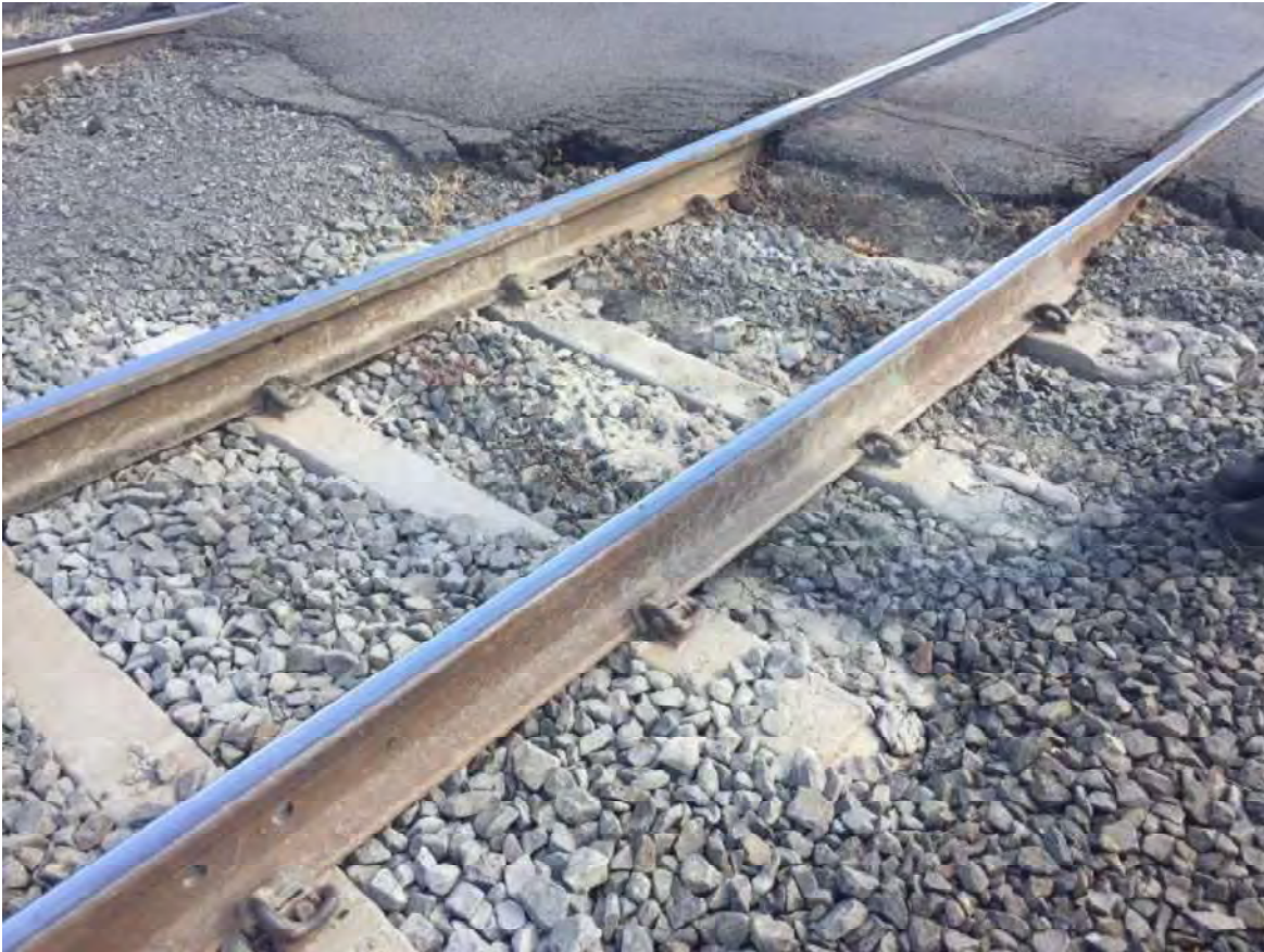
Figure 13: Impact of poor drainage on the condition of ballast
