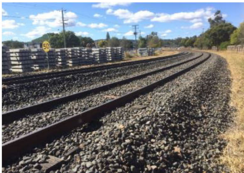
Figure 3: Poor track conditions in parts of the West Moreton system
