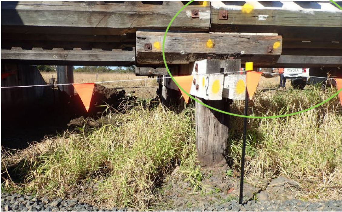
Figure 7: Timber-bridge structure in West Moreton system – support beams in poor condition
