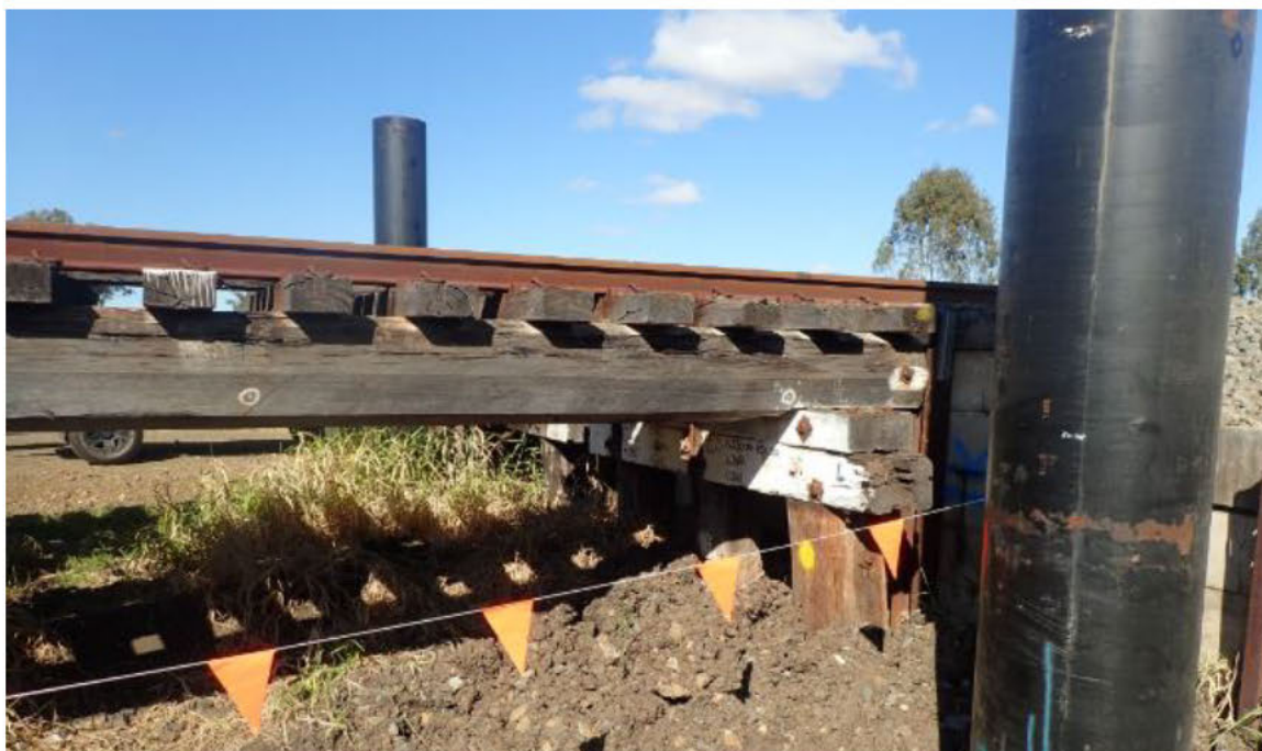
Figure 6: Timber-bridge structure in West Moreton system – failed girder (bearer)
