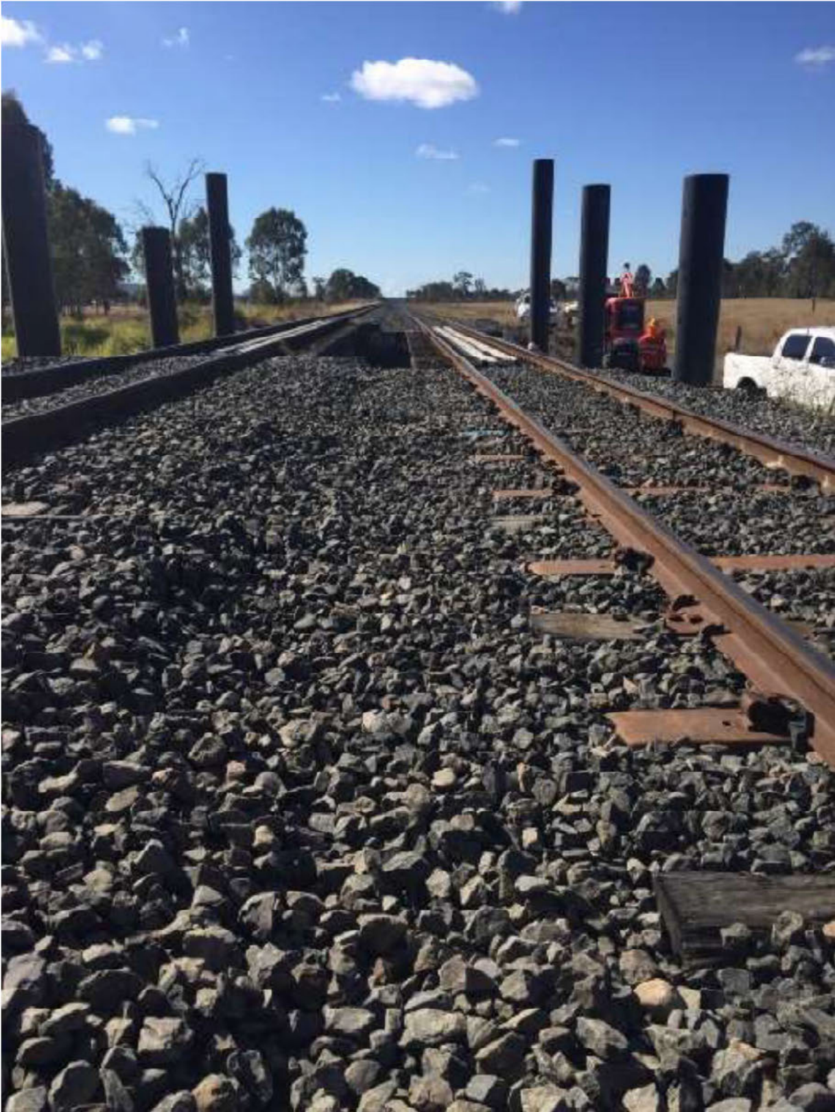
Figure 7: Use of a mix of steel and timber sleepers on parts of the West Moreton system
