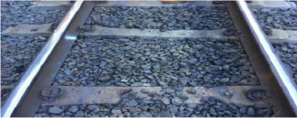
Figure 9: Skewed sleepers caused by excessive longitudinal forces
