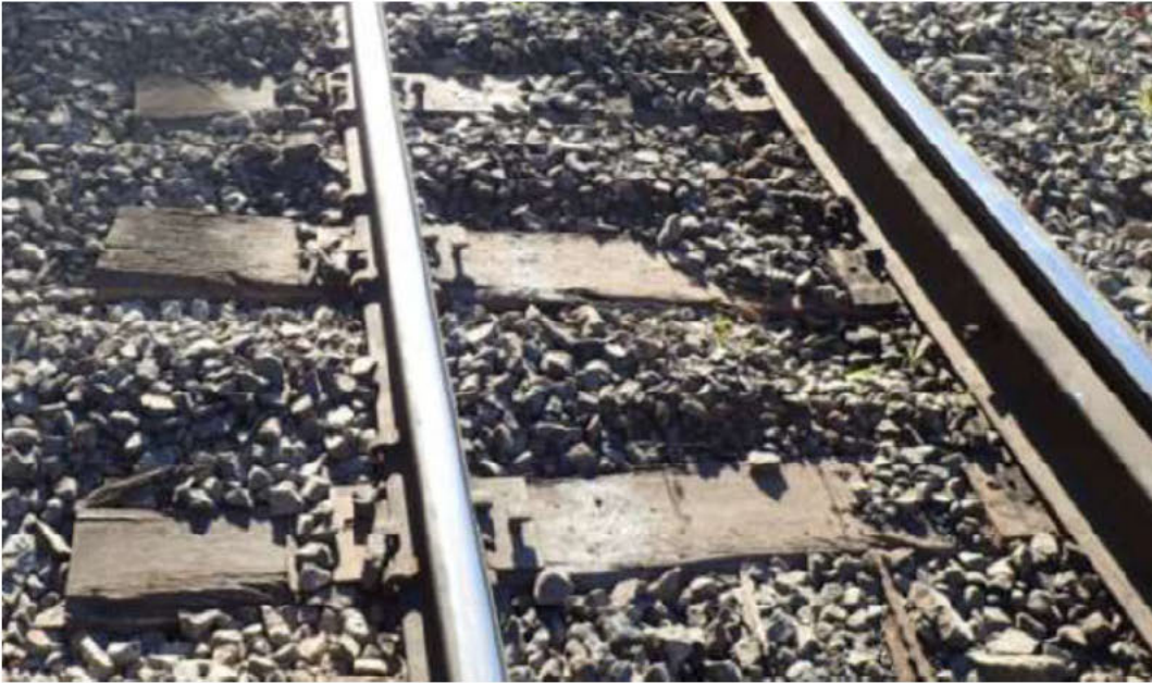
Figure 12: Skewed timber sleeper splintering
