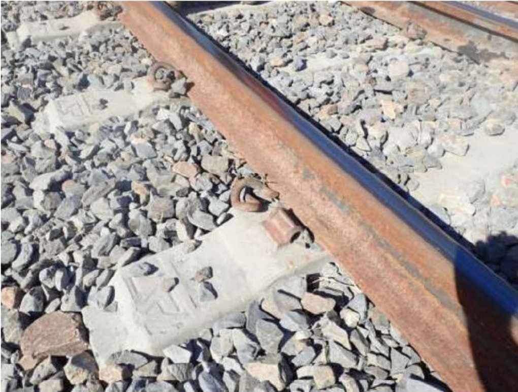
Figure 11: Missing sleeper clips and nylon
