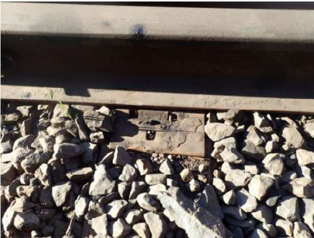
Figure 10: Missing dog spike
