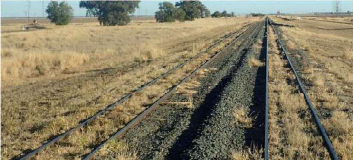
Figure 4: Dense vegetation growth through the track bed in parts of the track between Toowoomba and Miles, a symptom of the non-engineered formation characteristic of the West Moreton System
