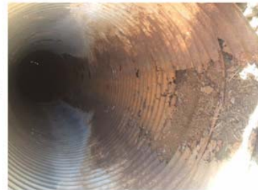
Corrugated metal culvert showing extensive corrosion
