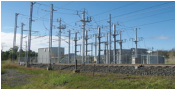
Track Sectioning Cabin at Westwood, part of the Wycarbah works.
