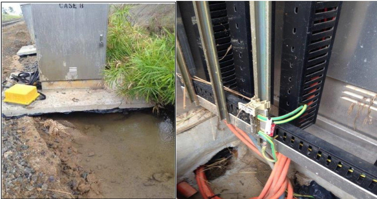
Figure 1: Damage to one of the signalling cabinets and the surrounding area at Mount Rainbow
