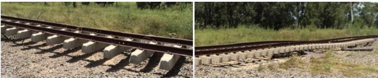
Figure 3: MSL-66 - ballast washout and formation loss between Earlsfield and Dakenba
