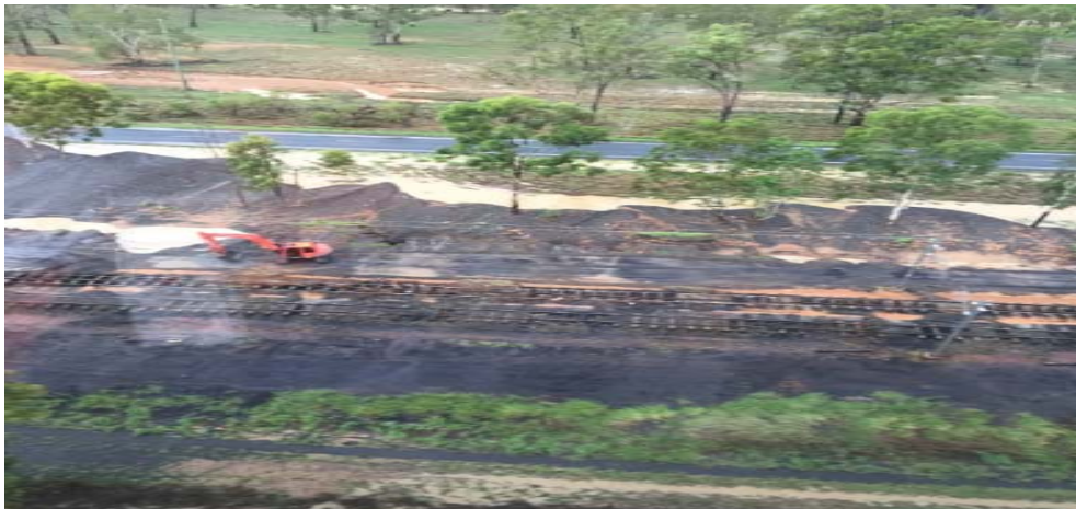
Figure 5 – Coppabella to Macarthur track washout
