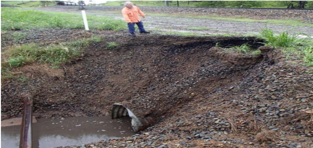
Figure 10 – disconnected pipe extension Daly Bay Junction
