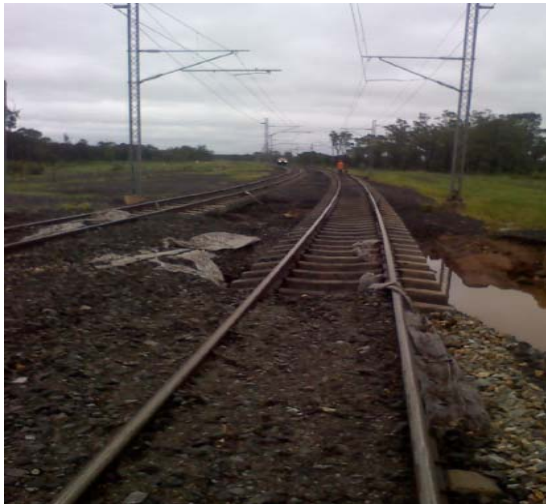
Figure 6 and 7 – Coppabella to Broadlea – sleeper scouring
