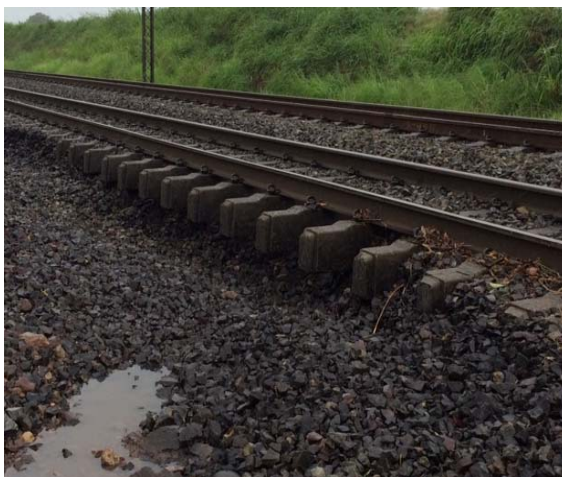
Figure 8 and 9 – Sleeper scouring at Yukan and Saraji
